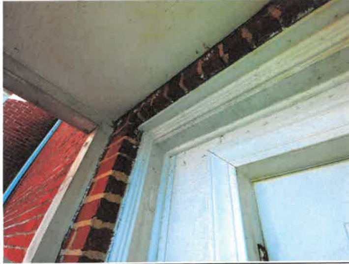
Window and door lintels on the back side of the Elliot Building were found to utilize lead-based paint.
