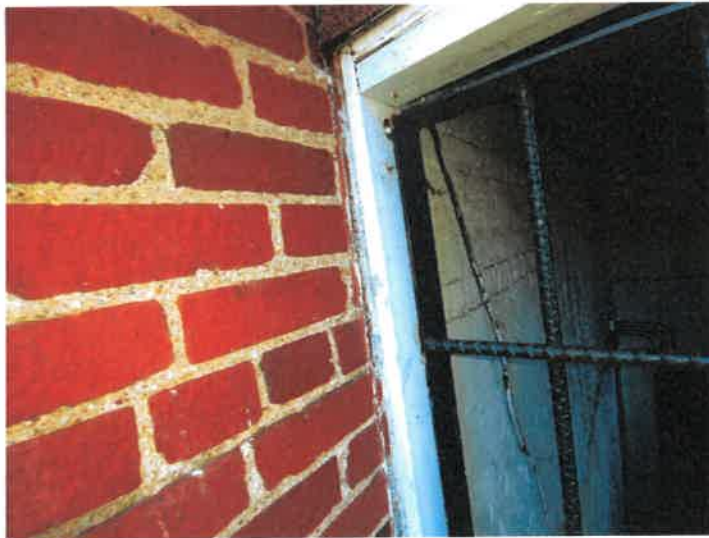
Painted wood door casings on the Plumb Alley side of the Elliot Building were found to utilize lead-based paint.
